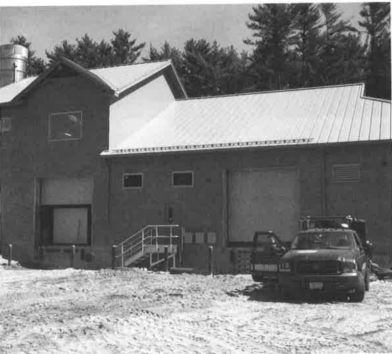
North Acton's Kennedy Marshall Treatment plant is on schedule for completion July 2009.
